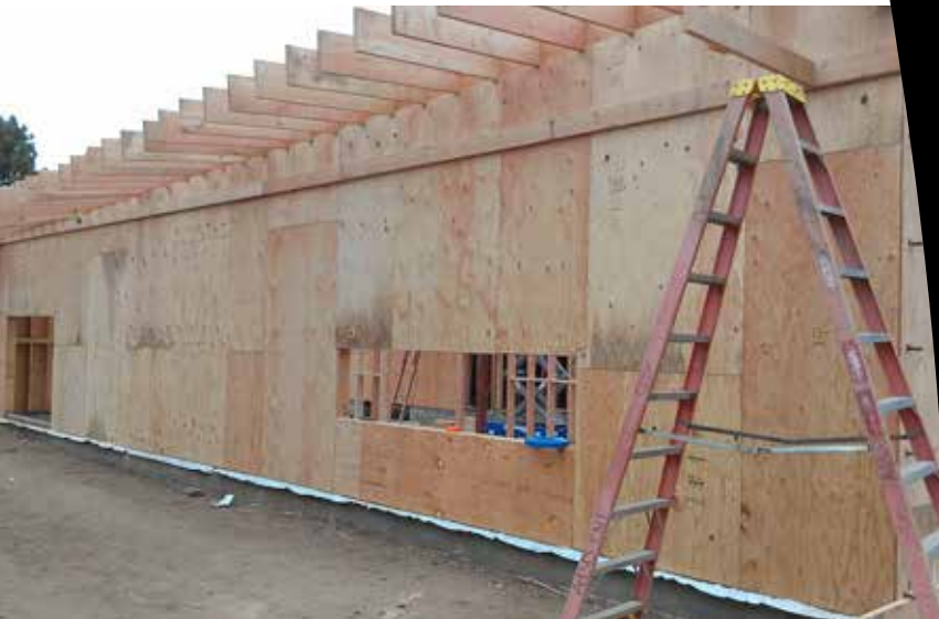
The Pico Branch Library under construction. All Roseburg Forest Products plywood used for sheathing at the Pico Branch was FSC certified.
